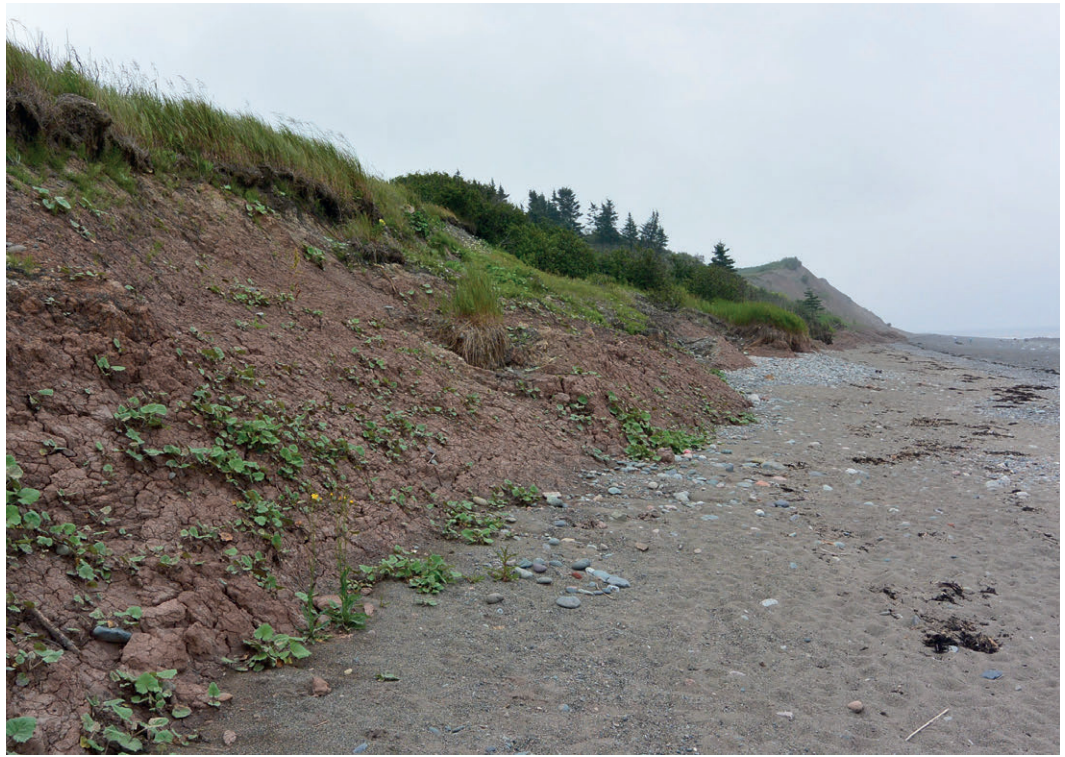
Figure 13: Shoreline erosion at Sand Cove Road in West Saint John (Photo: ACAP Saint John).
